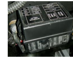
Fuse Box & Relays
