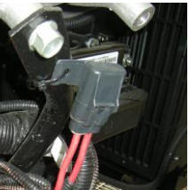
(Main 25A Fuse/holder) Primary key switch power via emergency switch.
