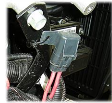
(Main 25A Fuse/holder) Primary key switch power via emergency switch.
