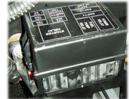
Fuse Box & Relays
