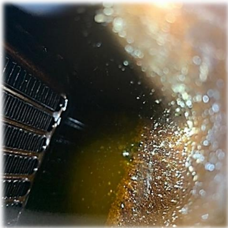
Clean Cooler with Condensation
