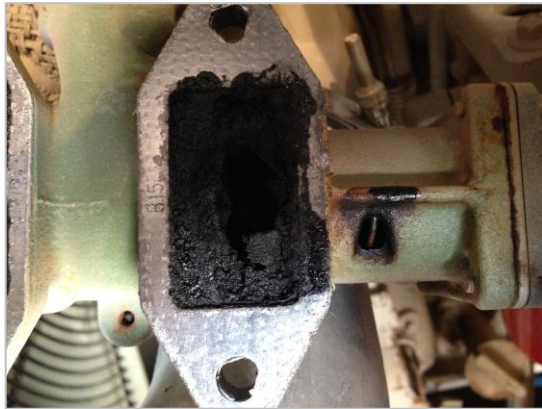
EGR VALVE CLOGGED
