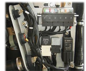
Fuse Box, Starter Relay, Fuel Feed Pump Relay, Pre-glow Relay
