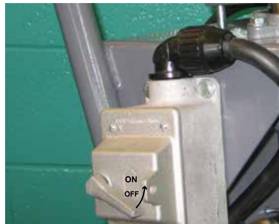
Figure 8. Electric Motor ON/OFF Switch
