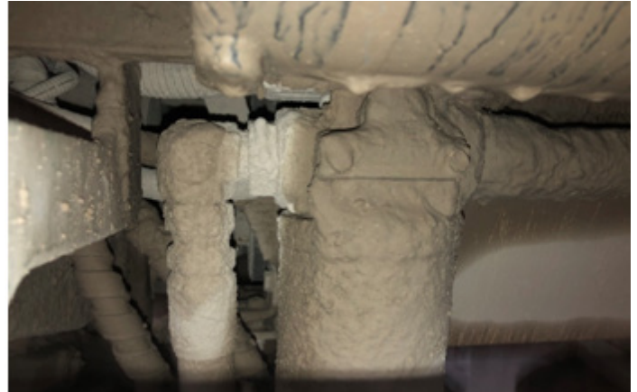
Slurry build up on hydraulic components may reduce cooling and increase chance of contamination during servicing.
